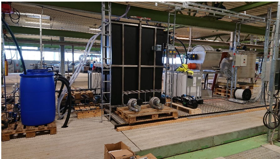
Figure. The Swedish pilot in place at Svedala wastewater treatment plant.
