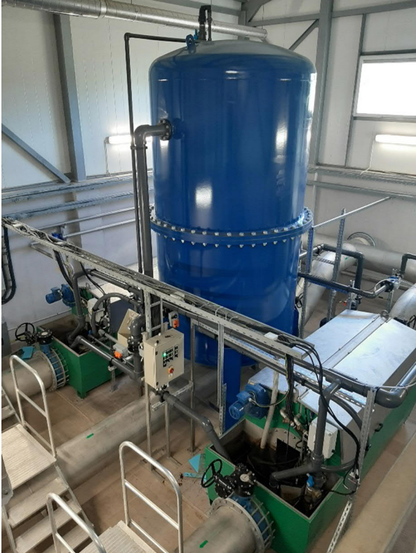
Figure 3-4: GAC filter photo in Kretinga WWTP
